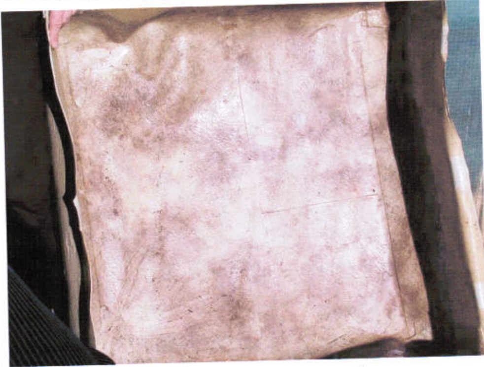
Image 1: Top of membrane without root ingress
